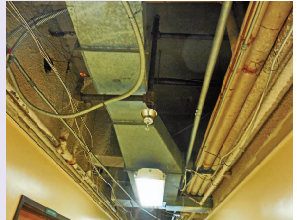
The downstairs classroom and hallway ceilings are exposed in order to repair/replace parts to the aging air conditioning throughout the building.
