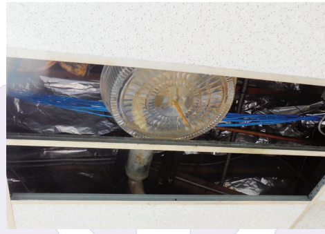
View of Betsuin office ceiling where water from the air conditioning condensation was accumulating in a sushi platter lid and dripping into containers below. [Article on page 5]
