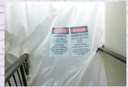
Warning signs sealing off the the lower level during the asbestos removal.
