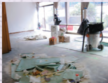
Emptied classrooms with no cabinets or flooring.
