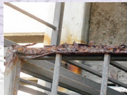
Top view of the security wrought iron fence that is rusting and flaking.
