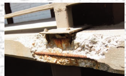
Crumbling concrete in the temple porch area.
